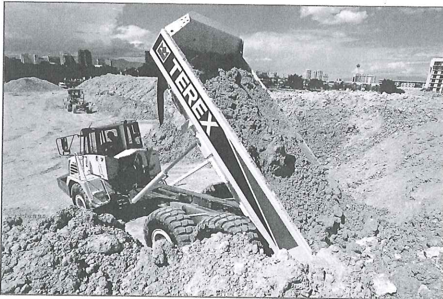
A Terex TA 30 haul truck dumps excavated material at the Crooked River Wetland Project.
