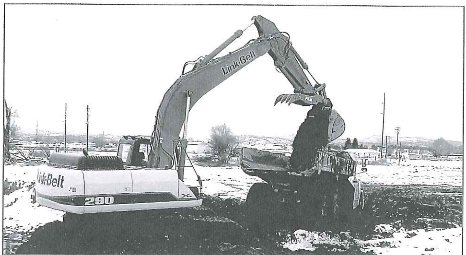
Using a Link-Belt 290X2 excavator and three Terex trucks rented from Triad Machinery, the City of Prineville moved nearly 80,000 yards of material to construct Phase II of its wetland project. Public Works Street Supervisor Scott Smith said the combination worked exceptionally well.
