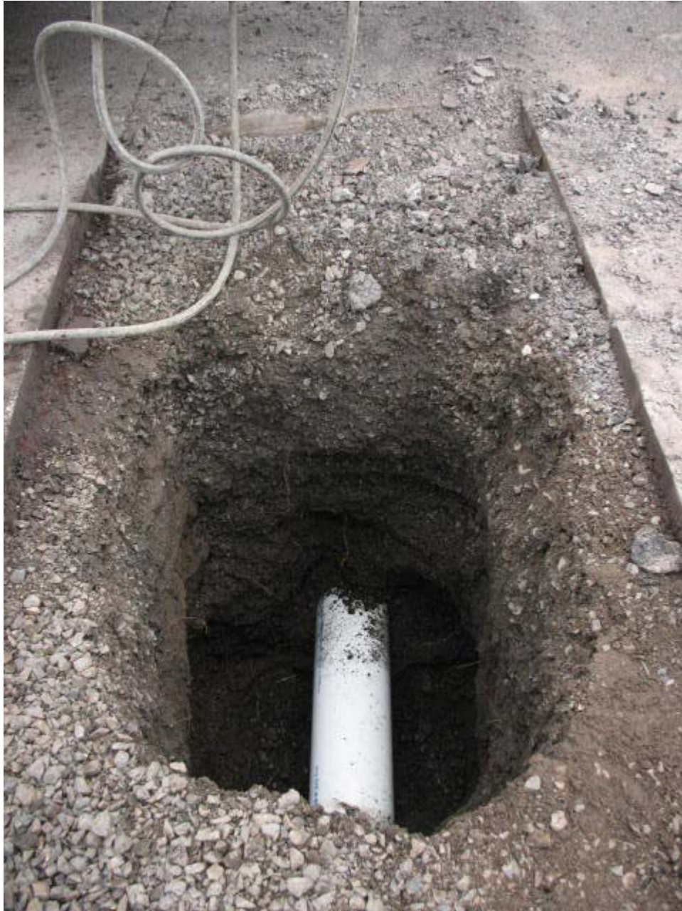
NW Corner of NW 4 th and NW Harwood 8" C-900 48" to top of pipe
